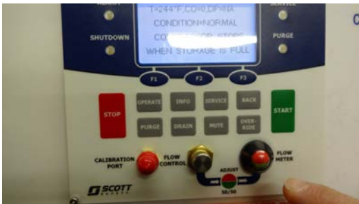
Ensure Flow Meter is 50/50 Red/Green Adjust with Flow Control
