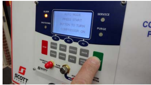
Push Start Compressor is now running
